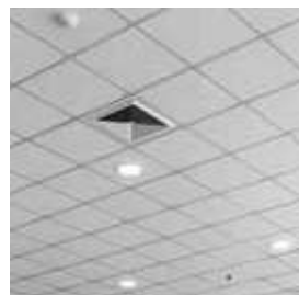
CEILING GRID FALSE CEILING
